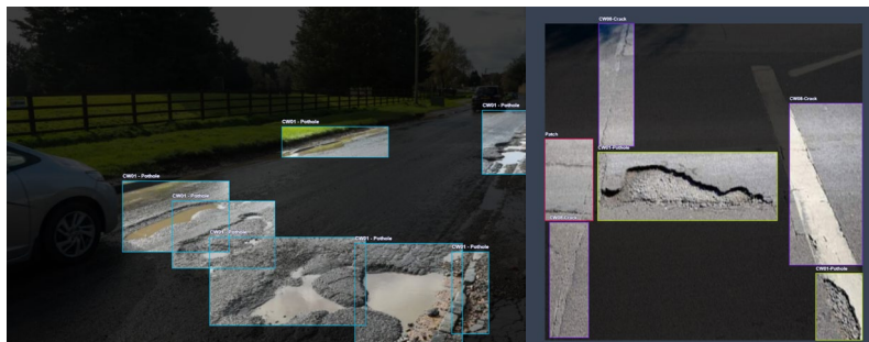
Figure 1: Labeled images showing potholes, cracks and patches.
